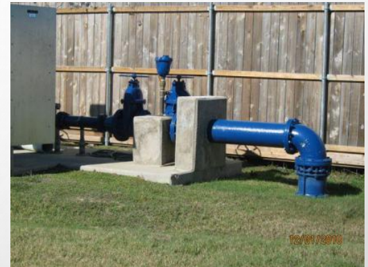
WHCRWA Surface Water Interconnect at Water Well No. 1 in Barkers Ridge Subdivision
